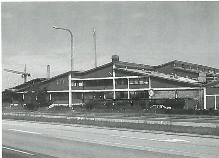
Martin's new factory to be. You won't be able recognise it from this photograph by the time the refurbishment is finished.
